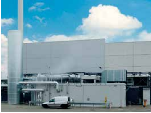
Danpower biomethane cogeneration plant on the site of the wind turbine blades producer Vestas Blades
